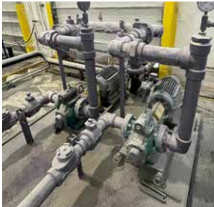
NOTOS® Multiple Screw Pump Application - mineral oil transfer from tank to manufacturing line.
