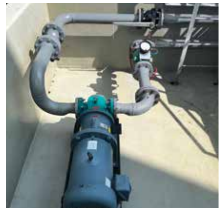
NOTOS® Same pump as above looking from motor side, just after commissioning.
