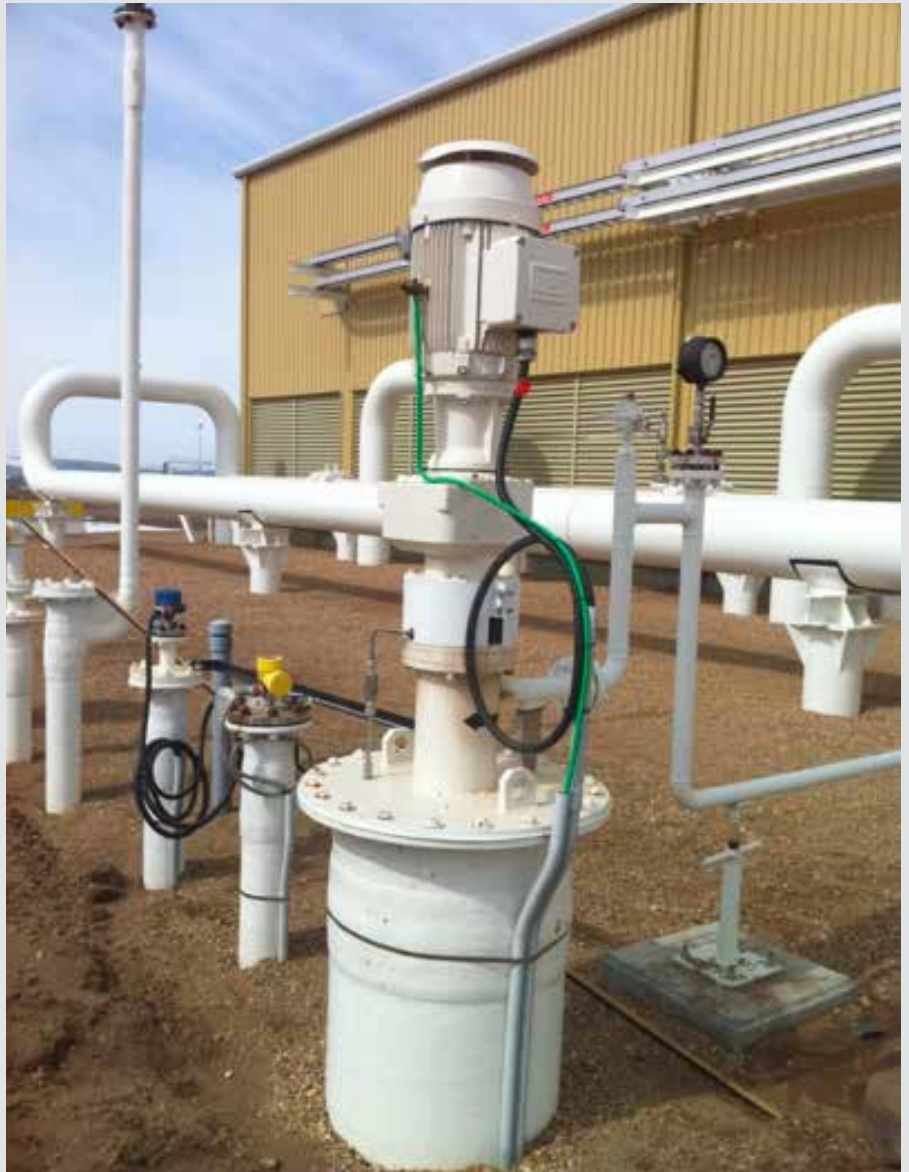
A need to reduce maintenance and simplify the transfer of oil from an underground tank back into the pipeline required NETZSCH to design and build a custom, 10-stage vertical progressing cavity sump pump to satisfy customer requirements.
