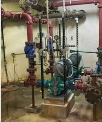
The City of Otsego WWTP installation of NETZSCH TORNADO® T2 Rotary Lobe Pumps.
