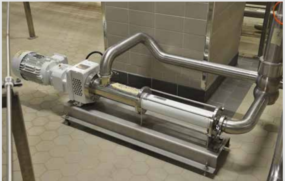
Liquid yeast dosing in the beer brewing process benefits from the precise metering capabilities of NETZSCH progressing cavity pumps (pumps 2 & 3).
