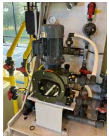
PERIPRO® C10/0.1 pump on sodium hypochlorite metering service skid
