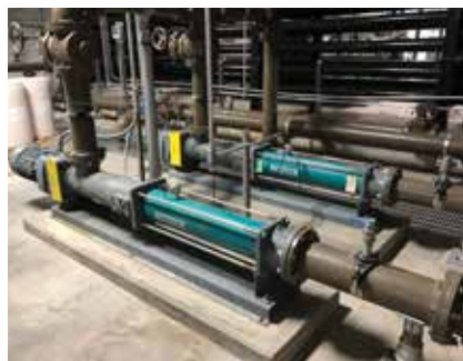
NEMO® BY Pumps transfer hydrolized food waste with extremely low pH
