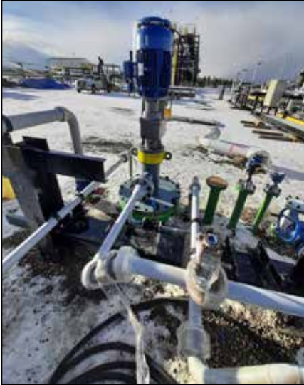
NETZSCH NEMO® BT is installed on top of the drum which is below grade.
