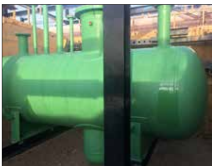
Typical horizontal knockout drum
