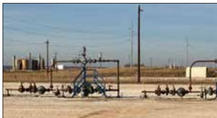
Multipad well site employing the gas lift method
