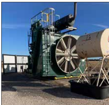
Compressor used to re-inject the gas into the well bore to force the fluids to the surface.
