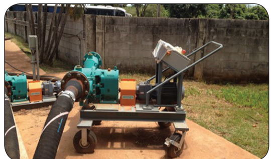
Trolley mounted TORNADO® T1 Rotary Lobe Pump transferring sewage
