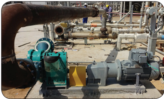
TORNADO® T1 transferring oily sludge
