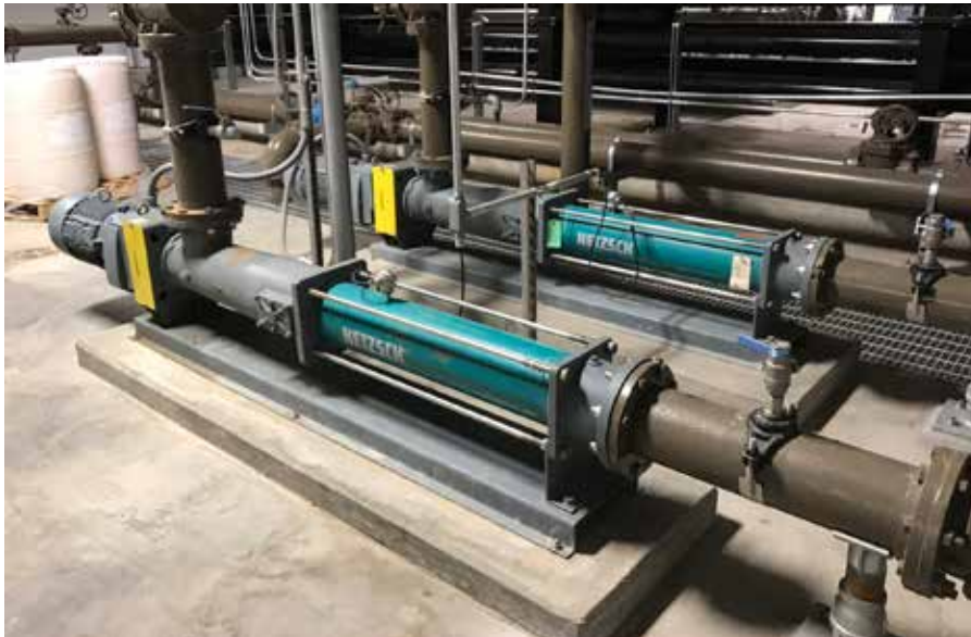
NETZSCH NEMO® 090 BY pumps in the Boiler Building transfer hydrolyzed food waste with extremely low pH product with 5% solids.
