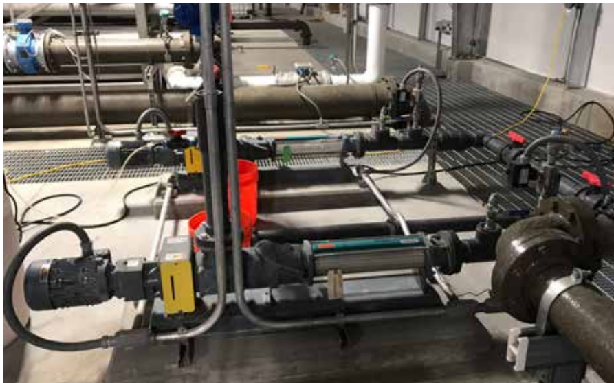
NETZSCH NEMO® FSIP® pumps in the boiler building to pump grease trap waste from restaurants and bacon grease from local bacon manufacturer to convey product to the digesters.
