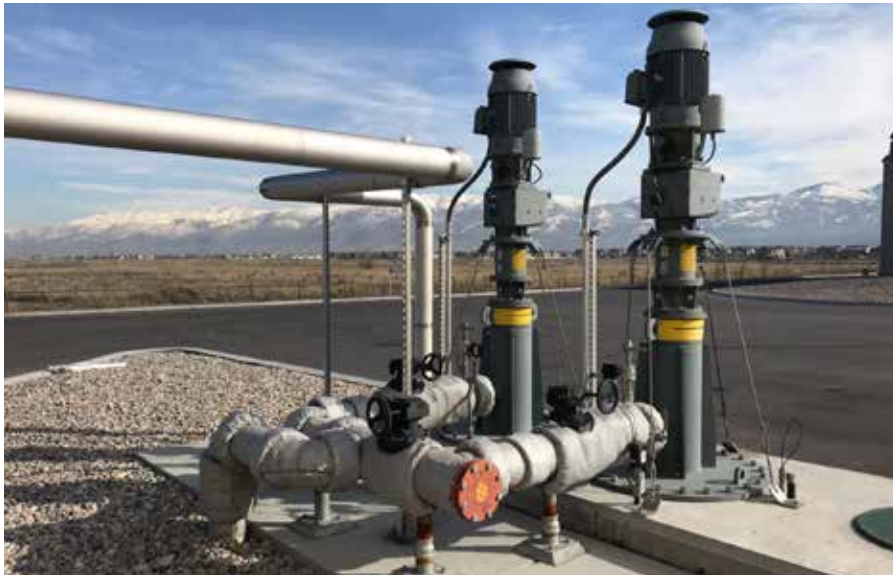
NETZSCH NEMO® BT pumps for hydrolysis feed at liquid wasterreceiving building (liquids, de-packaged waste from dog food, food products, fruits, grocery waste, and produce.
