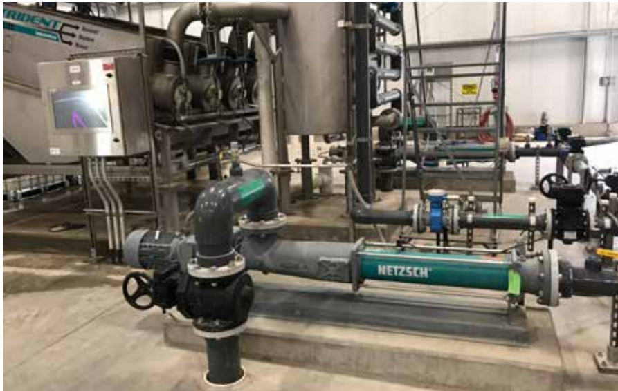
NETZSCH NEMO® FSIP® pumps in the chemical recovery building pumping post struvite production to water removal
