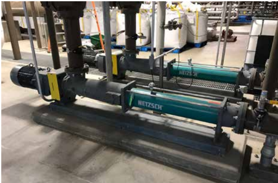
NETZSCH NEMO® 090 BY pumps in the Boiler Building provide a feed to the Struvite production.
