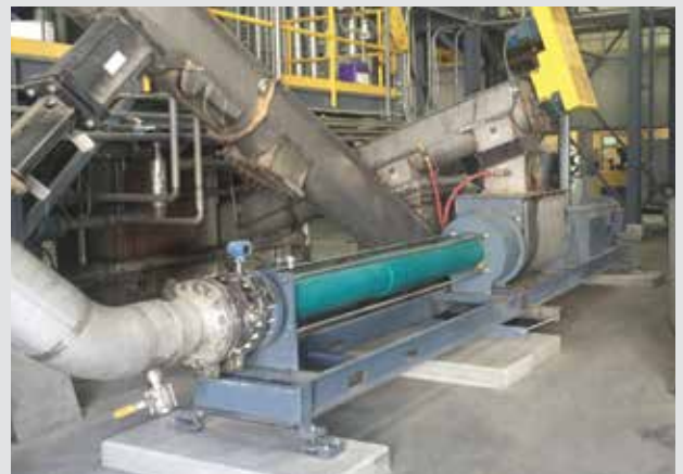
The NETZSCH NEMO® SF Progressing Cavity Pump in the Pacific Ethanol facility has a customized system to move wet cake.
