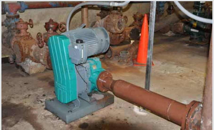
NETZSCH TORNADO® T2 Rotary Lobe Pump seen in operations in sludge transfer line.
