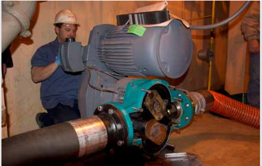
A Veolia maintenance engineer checking the NETZSCH TORNADO® T2 Rotary Lobe Pump during routine maintenance. Note the easy access to rotors from front of the pump.
