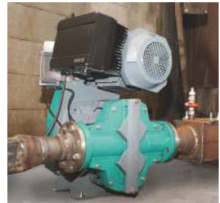
Pumping liquid manure in a biogas plant
