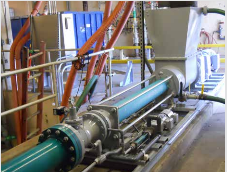
The filter cake pump system is designed to transfer the cake by rotation of a metal rotor within a compressible stator.
