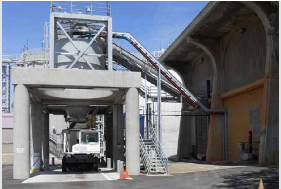
Storage hopper with collection truck.
